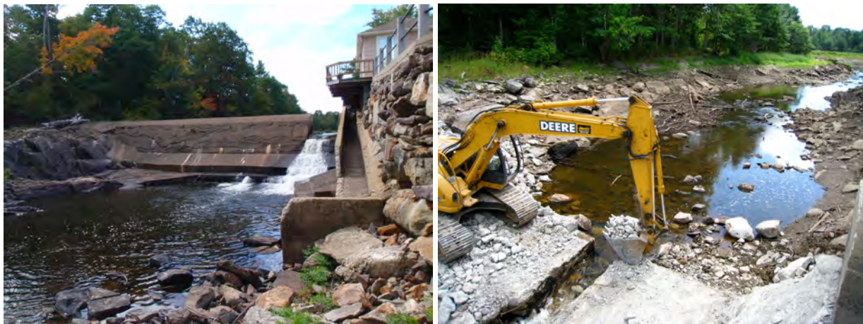
Figure 3. The Winterport Dam on Marsh Stream, Penobscot River basin, Maine showing the dam removal from downstream (left) and the upstream drawdown of the reservoir in 2010. The removal
